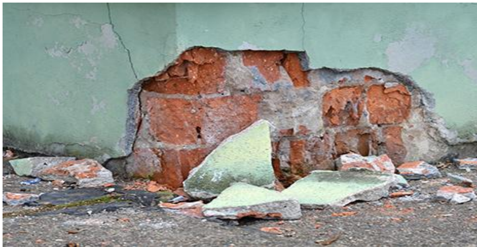
Figure III.11. Swelling of the masonry. Source : (Mur Humide, 2024)
