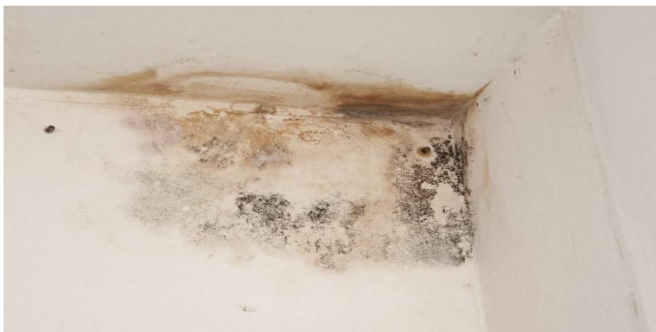
Figure III.12. Mold on a wall. Source : (Humidité-Expert, 2024)
