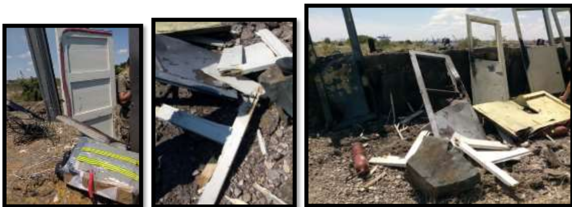
Figure 8. DES applied at various points on wooden and metal doors of different types;
