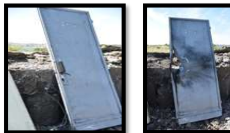
Figure 5. Cutting with DES flexible creating BLADE type breaches, made of DEMEX type plastic explosive (1150g / ml with a length of 140mm) fixed on the lamella from a sintered copper mixture, fixed on a metal door handle.
