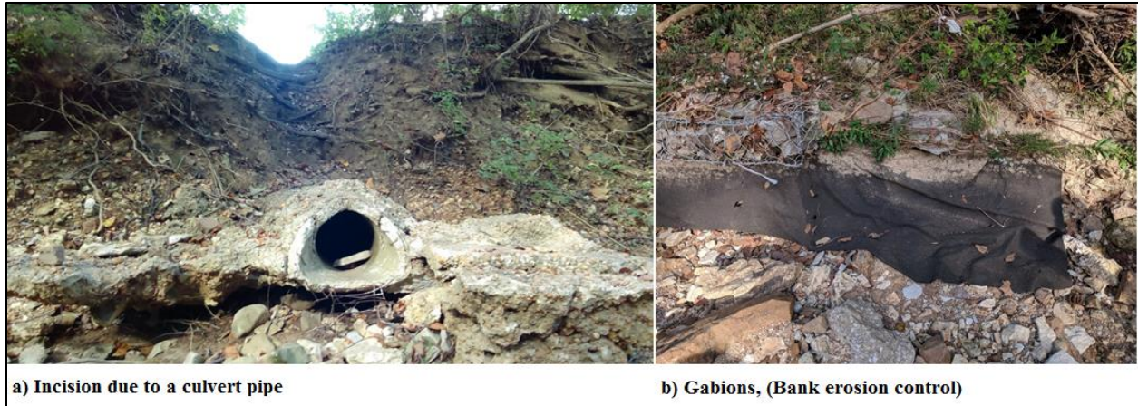
Figure 5. (a) Incision formed on the bank due to a culvert pipe. (b) Gabions for bank erosion control with geotextile to prevent smaller particles from being eroded from under the rocks.
