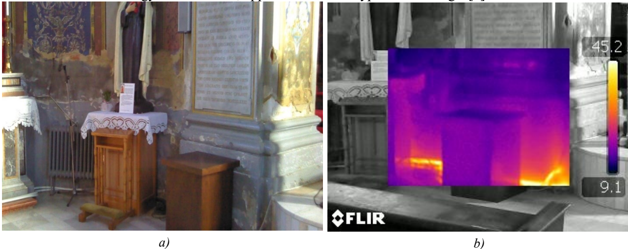
Figure 1 a) Degradation due to the appearance of condensation at the base
