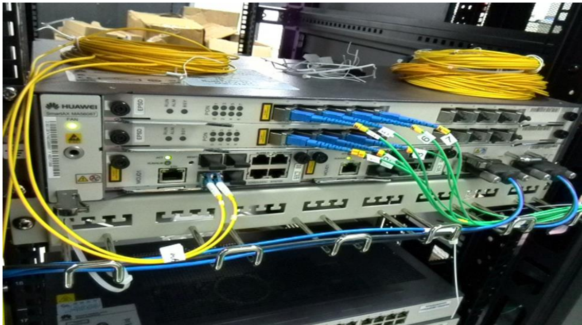
Fig. 4.1. OLT connected with optical fiber and modulators
