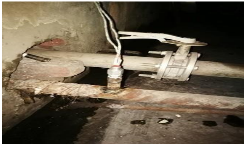
Fig- 4.2 Connection of sensor probes in condensate water pipe
