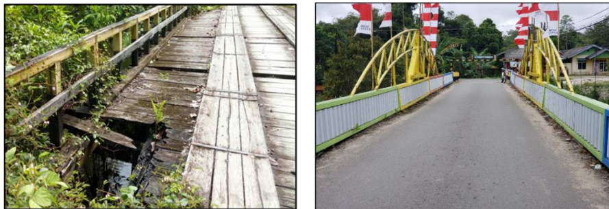
Figure 4. Bridge Condition Before and After Maintenance by Innovation
